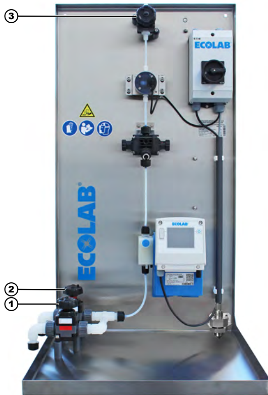
Fig. 5: Flushing valve and maintenance valves
