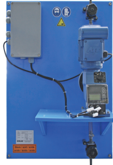
1 EMP III Pumpe
